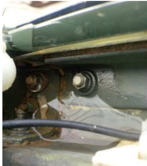
Clogged Drain Hole In Window Frame Assembly:
