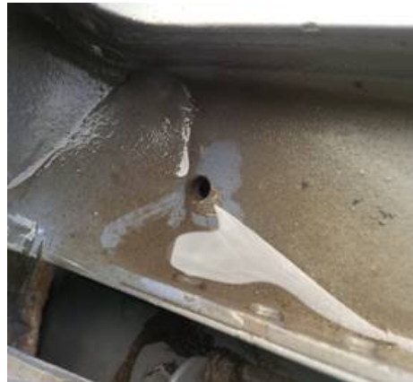
Clogged Drain Holes in Window Sill (Structure):
