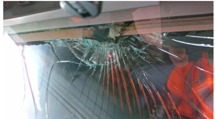
View from inside, upper aft bus bar area, on ship
