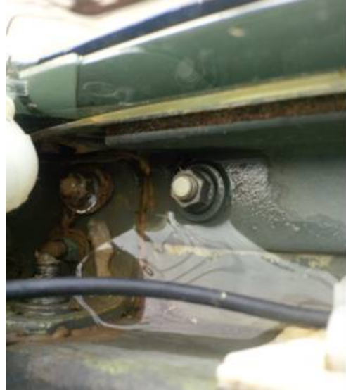
Clogged Drain Hole In Window Frame Assembly:
