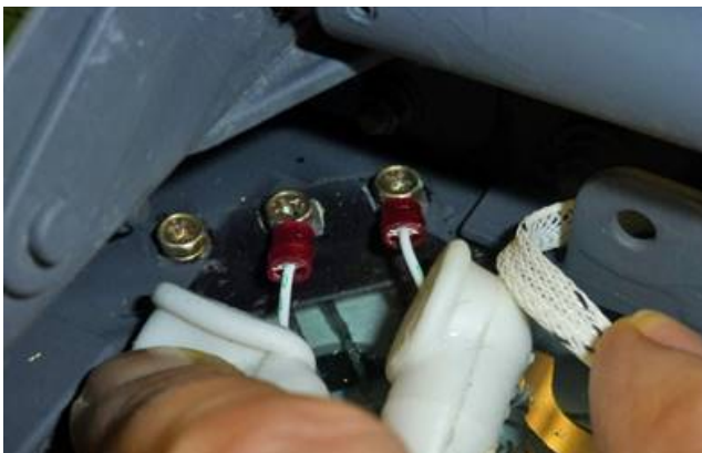
Clean Terminals, Ruber Boots Installed and Not Damaged:
