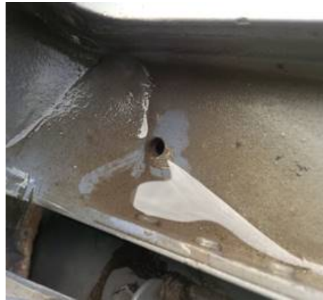
Clogged Drain Holes in Window Sill (Structure):
