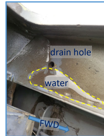
Water accumulation in window frame sill due to plugged drain hole.
