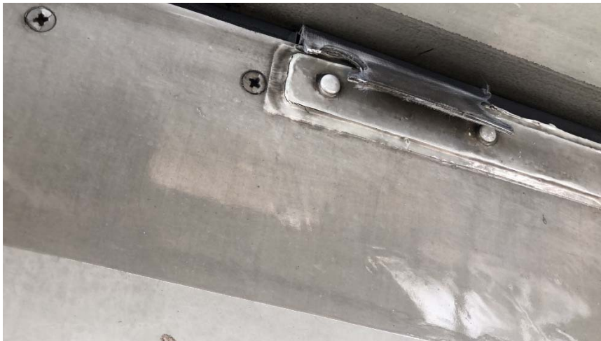
6# I/B BULB SEAL DAMAGE.
